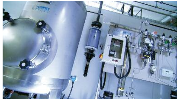
Figure 35: HPW water treatment plant
