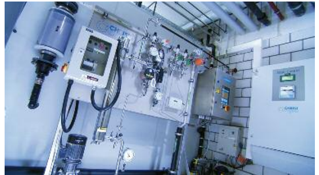
Figure 36: HPW water treatment plant
